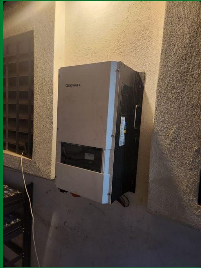
PPPIF-FUNDED SOLAR INVERTER
